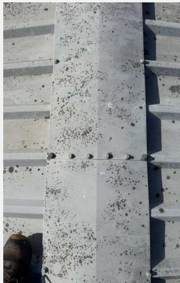
RIDGE CAPPING JOINT - FIXINGS IN PLACE; DIRT, LICHEN AND MOSS ON THE CAPPING
