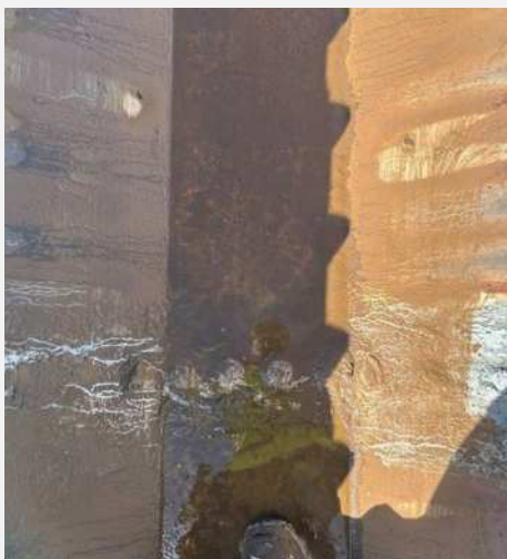
VALLEY GUTTER JOINT - CORRODED JOINT BOLTS; FAILED SEAL; ALGAE AND STANDING WATER AT THE JOINT
