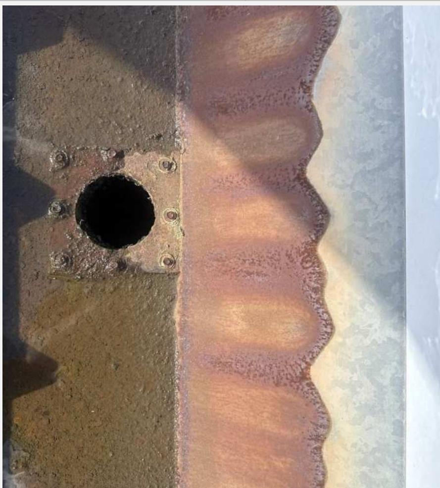
EXTERNAL PERIMETER GUTTER OUTLET - NO LEAF GUARD; CORRODED FLANGE BOLTS; RUST AND SILT TO THE GUTTER SOLE AND HEAVY RUST STAINING TO THE SIDEWALL
