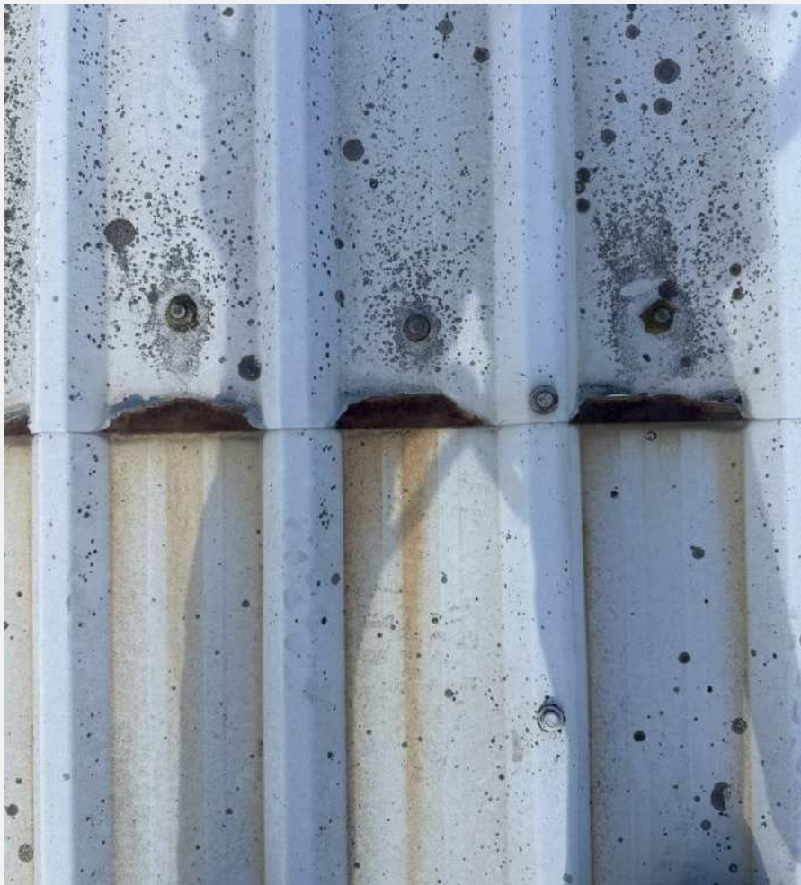
SHEET END LAP - COATING DELAMINATION AND CUT-EDGE CORROSION ALONG THE LAP; LICHEN AND DIRT ON THE SHEETS; RUST STAINING BELOW THE LAP
