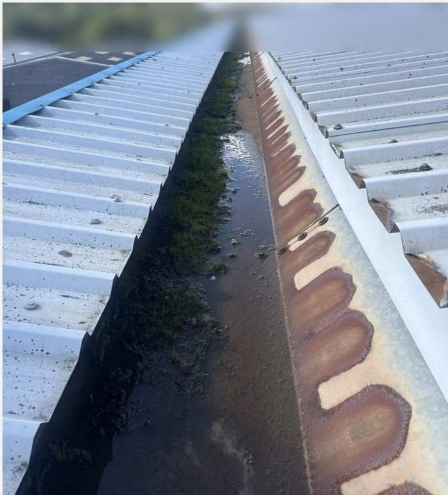
EXTERNAL PERIMETER GUTTER RUN - SILT, GRASS AND STANDING WATER IN THE GUTTER SOLE; HEAVY RUST STAINING ALONG THE SIDEWALL
