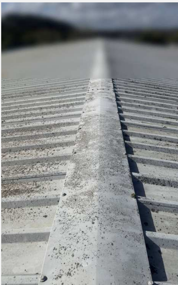
RIDGE CAPPING ALONG THE ROOF - CONTINUOUS AND FIXED; DIRT, LICHEN AND MOSS ON THE CAPPING
